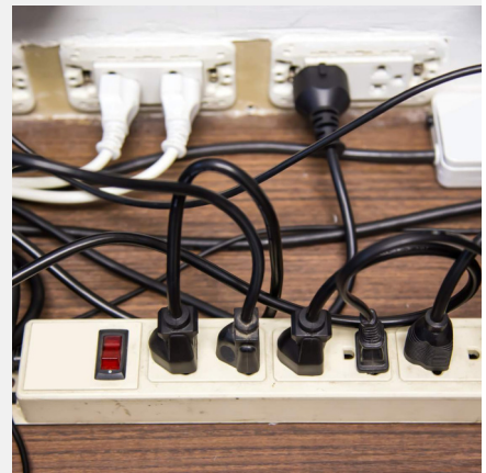
Electrical equipment used the wrong way
